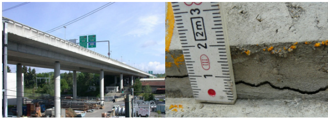
Figure 11. Viaduct Weyermannshaus, concrete crack (SWITZERLAND)
